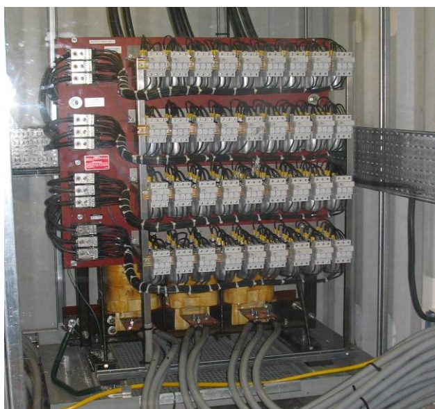
Fig. 18. One of two 750kW Lineator™ units installed on each group of 750kW combined thruster and pump load
